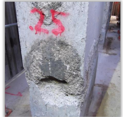
Concrete that has been affected by sulfate attack
