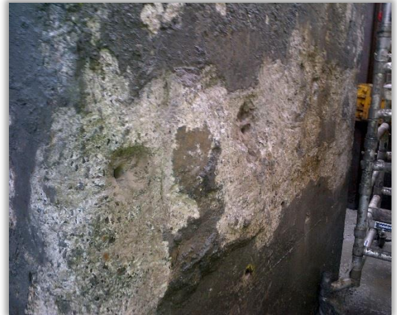
Concrete corrosion – subjected to sulfate (thaumasite) attack
